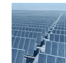
Benban 50MW PV IPP
