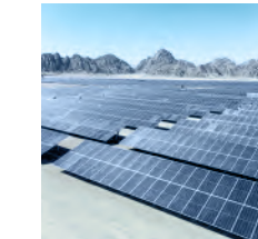
Sharm El Sheikh Solar Power Plant
