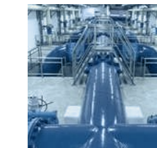
Abou Qoueiqal Water Treatment Plant
