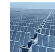
Benban 50MW PV IPP
